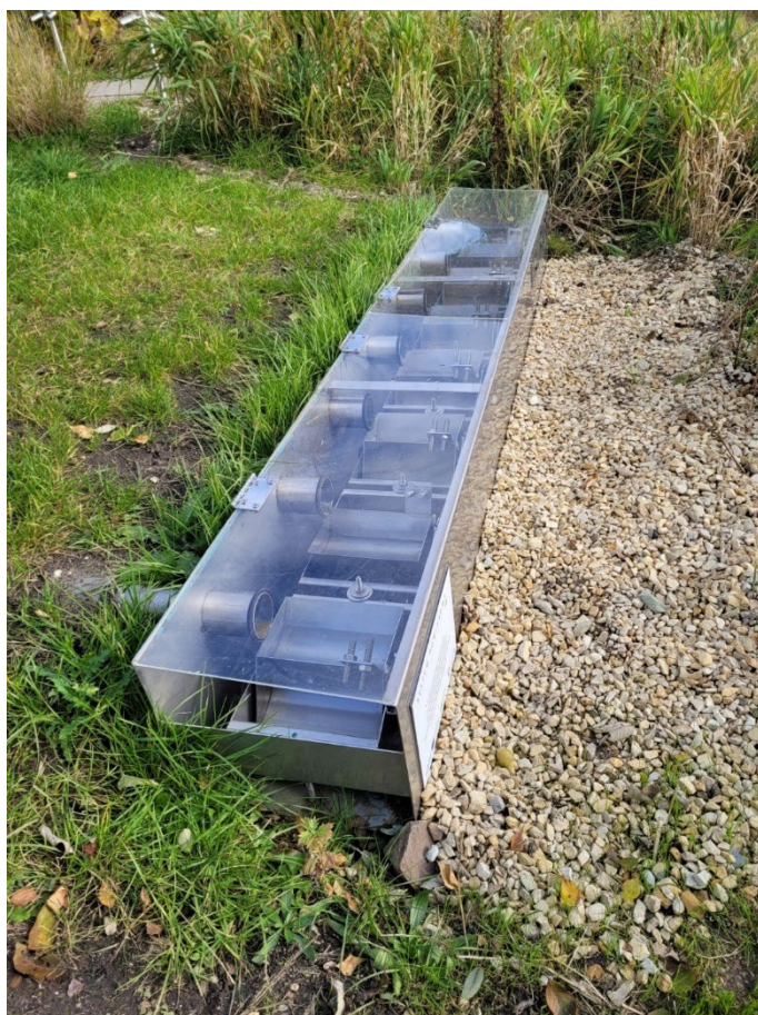
Photo 3: Pilot installation in Jaworzno - tipping bucket flow measurement system
