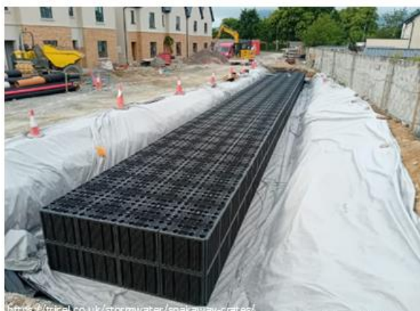
https://tricol.co.uk/stormwater/soakaway-crates/ Geocellular soakaway crate system at Residential development in Killarney (Ireland)
