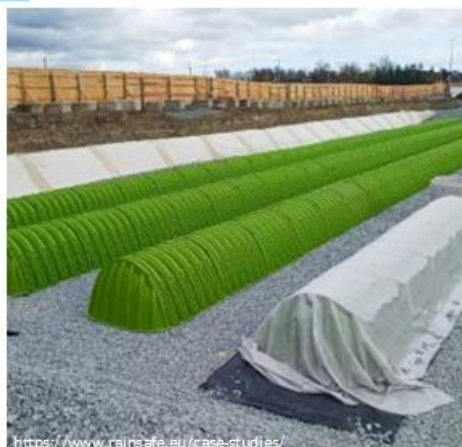
https://www.rainsafe.eu/case-studies/ Large Soakaway System for Sustainable Stormwater Management at Griffeen Community College (Ireland).
