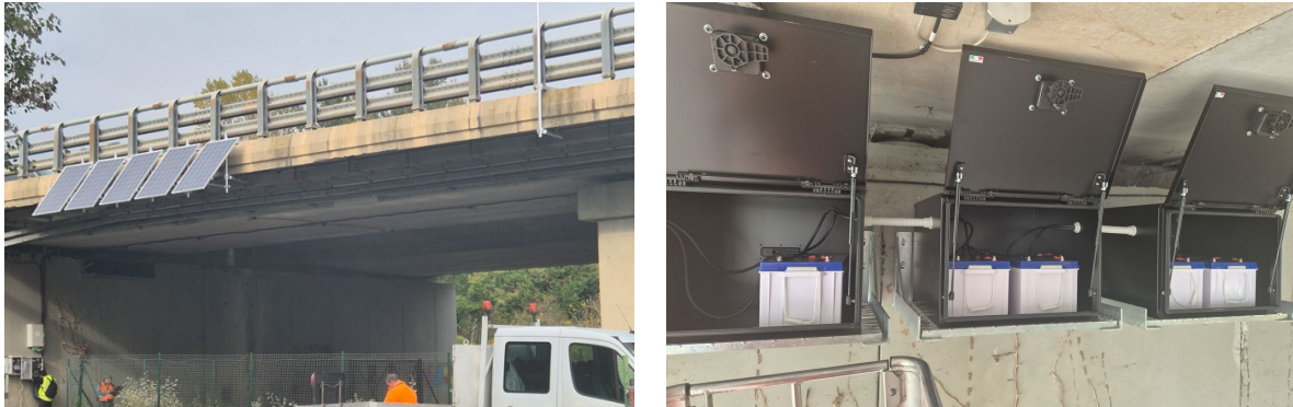
Figure 21. Power supply system on Sant'Ambrogio bridge
