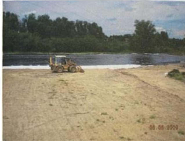
Figure 3. Placement of a waterproof layer and profiling of the layer in 2009-2010. Source [2]
