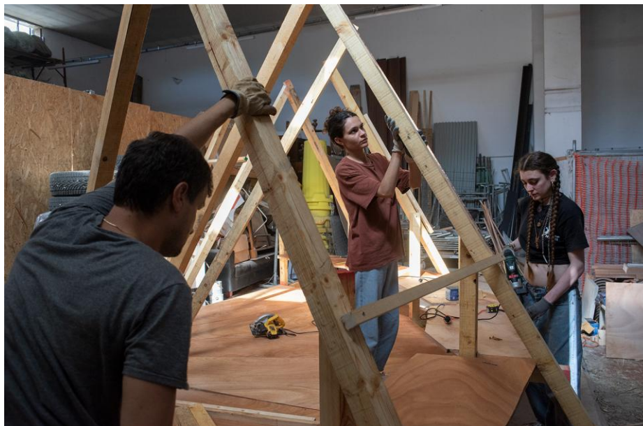
Co-design lab in Ferrara, where community members built timber structures for shading, demonstrating how tactical urbanism thrives on hands-on participation and shared ownership. Credits: Matteo Cattabriga
