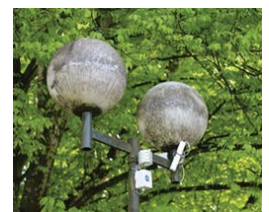
Climate sensors installed on street lamps
