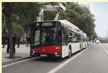
Charging infrastructure at bus stop
