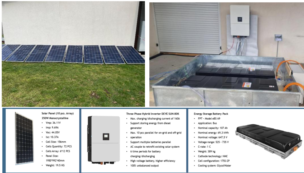
Figure 7: Key components of the BESS system: PV panels, inverter and second-life battery pack.
