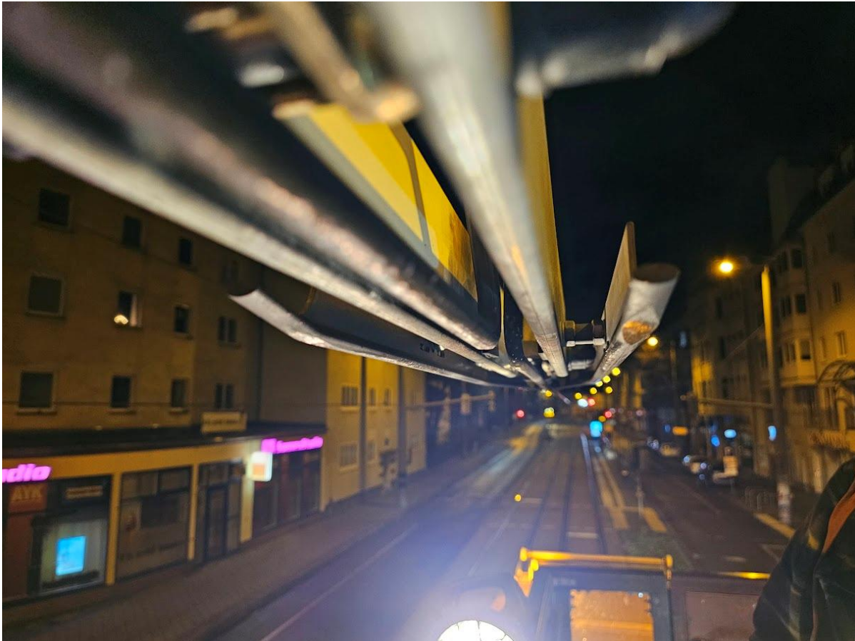
Figure 9 A misadjusted section insulator
