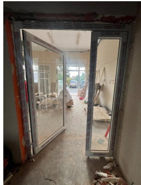
Figure 8 Multicentre's renovation – view from the carpentry room to open-space. Source: Municipality of Brzeg Dolny.
