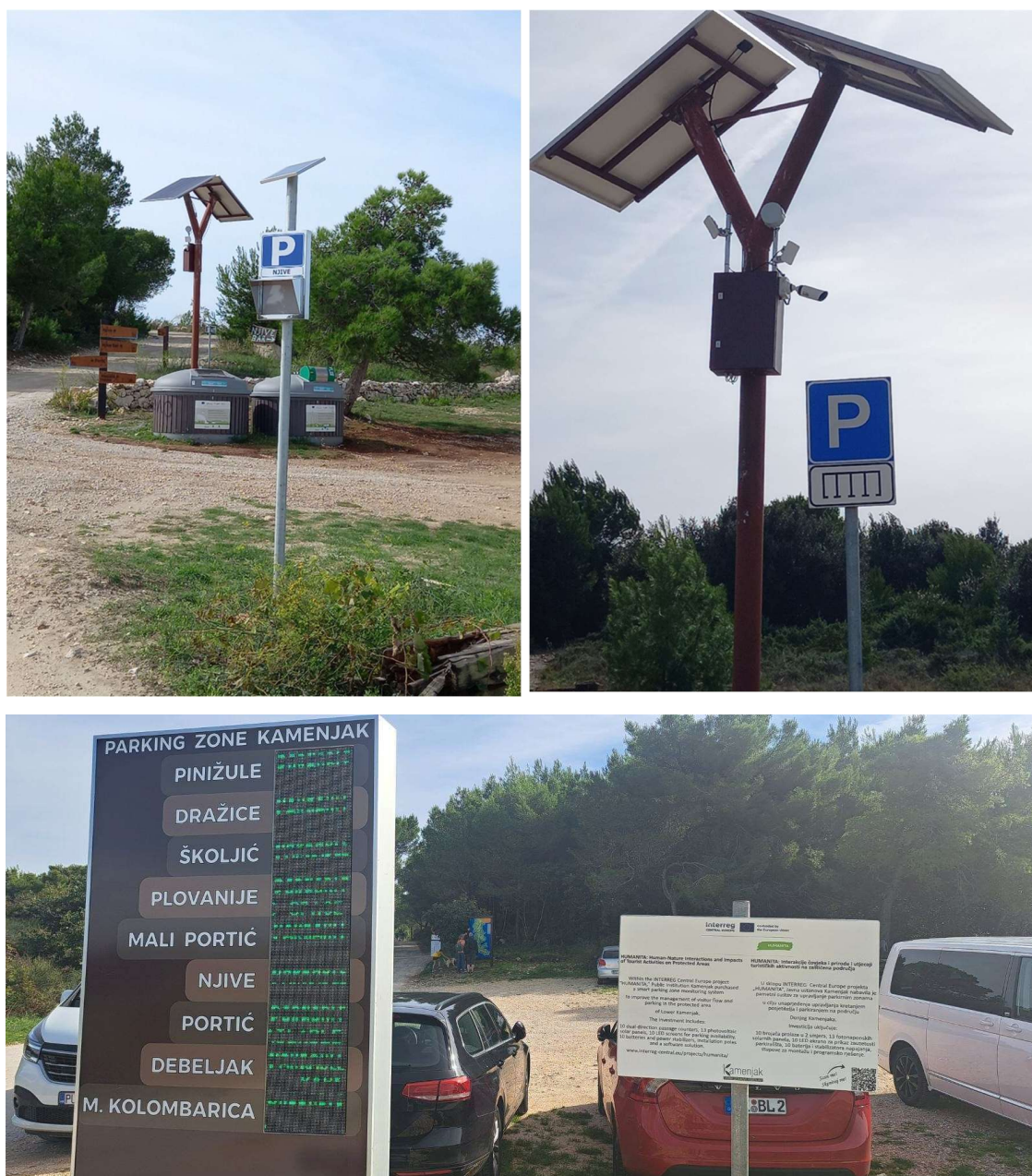
Figure 1. Installation of LED panels and solar-powered cameras at the entrance of the Lower Kamenjak area. The LED panels provide real-time information about parking zone availability, while the cameras monitor vehicle entry and exit using laser technology, ensuring efficient visitor management.
