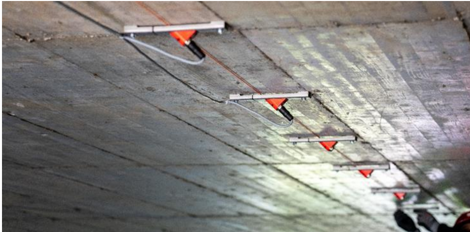
Figure 3 ST-504 sensors installed on the deck of a bridge
