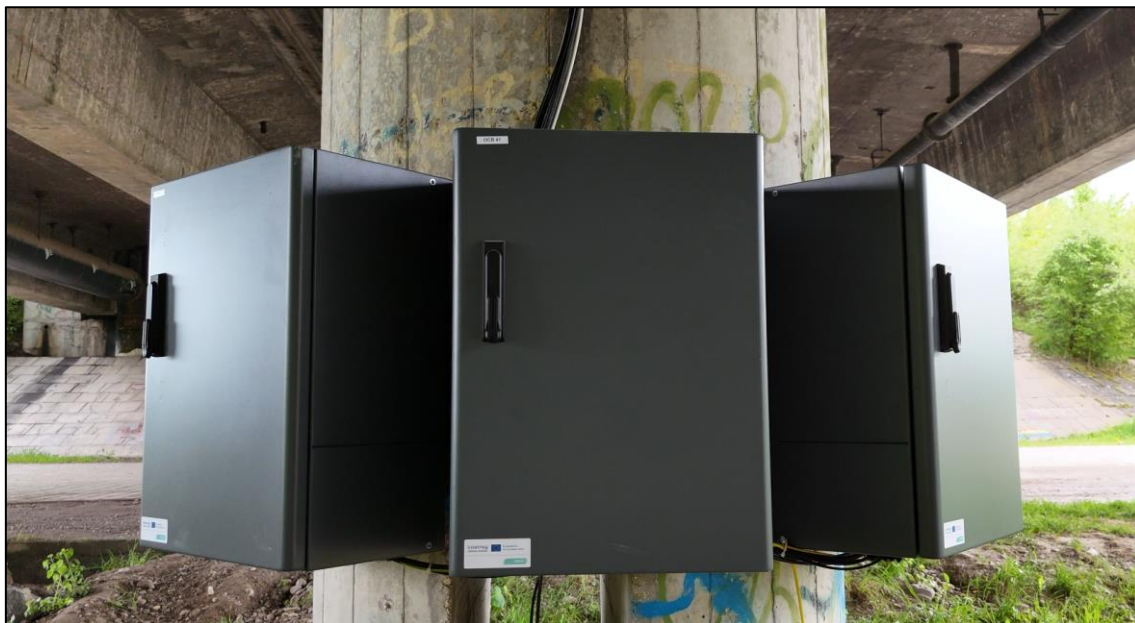
Figure 10: Cabinets of the system - one cabinet contains the electronic components of the bridge WIM system, another one contains the components of the SHM system, the last one is an electrical cabinet (Source: Cestel).
