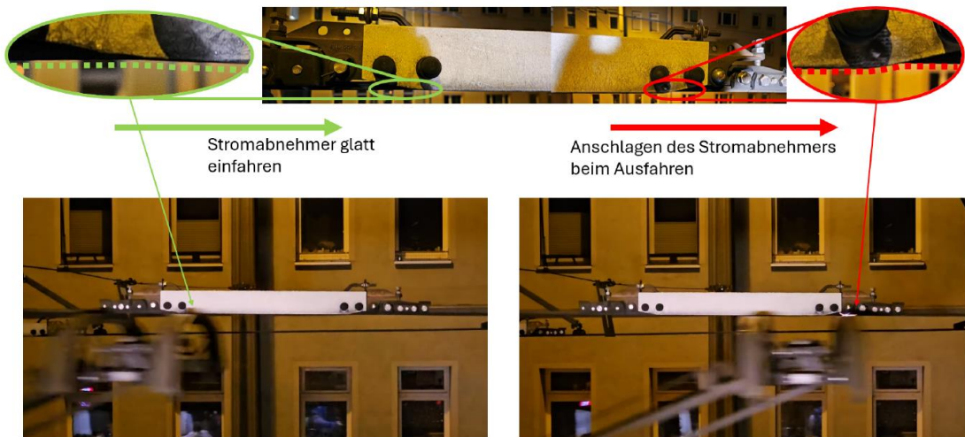
Figure 7: Current collector retracts smoothly and hits the section insulator when extending, no arcing when retracting, but arcing when extending
