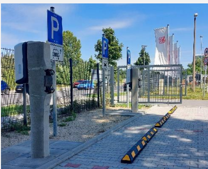
Figure 25 Recycled concrete polls. Source: Deutsche Bahn
