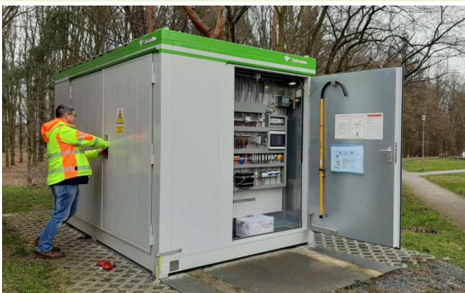
Figure 15. Buffer storage in Pilsen. Source: Interreg EfficienCE publication.
