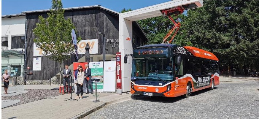
Figure 14. Opportunity "pantograph" charging station in Maribor. Source: https://programme2014-20.interreg-central.eu/
