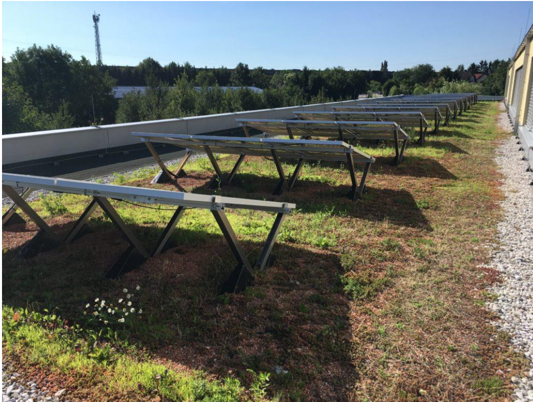
Figure 30: Extensive Green Roof combined with photovoltaics on a kindergarten, Bad Vöslau 42
