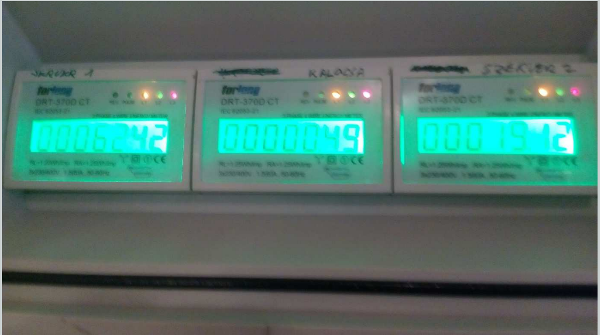
Server electricity consumption meter
