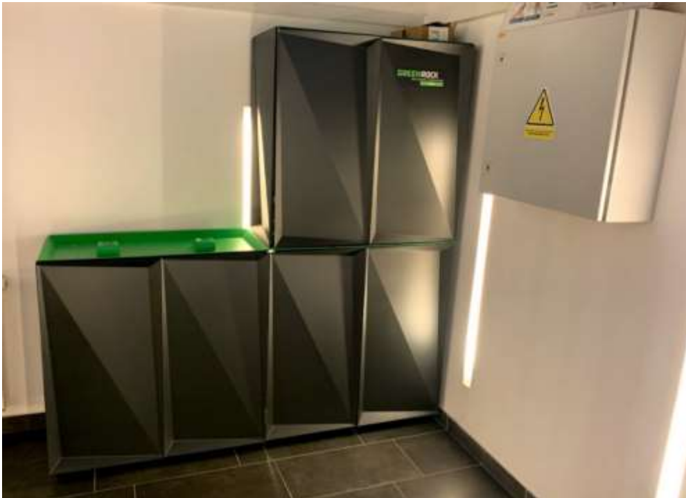
Figure : The storage (battery system) is placed in the premises of the Bracak Manor, in the basement next to the stairs (Source: REGEA 2021)
