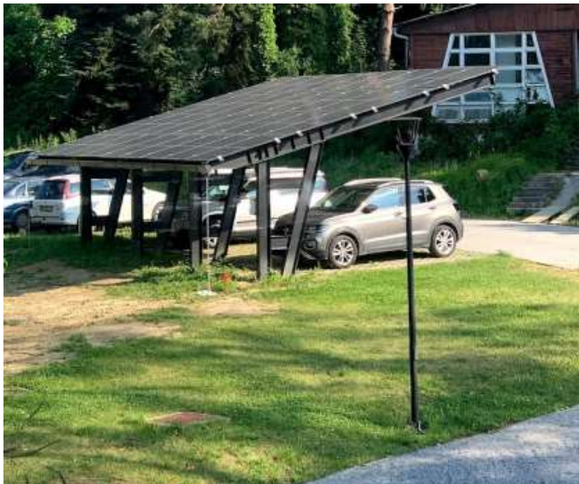
Figure: Installed photovoltaic modules Source: REGEA
