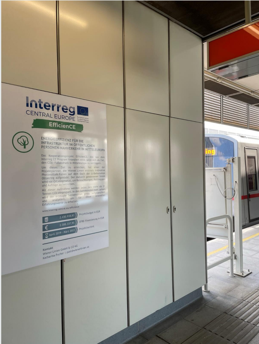
Figure 4: Branding of the PV-System on the metro stations public platform, Copyright Wiener Linien GmbH & Co KG
