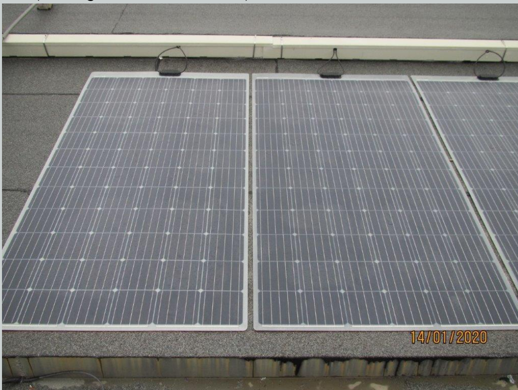
Figure 1: Photovoltaic foils bonded to the ground (01-2020), Copyright Wiener Linien GmbH & Co KG
