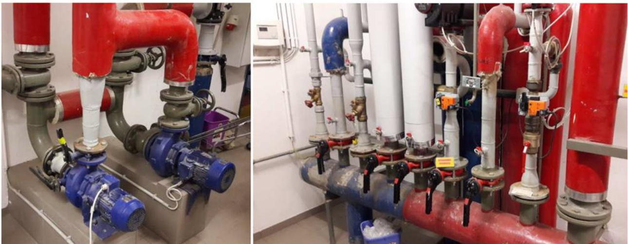
Figure 1: Investment activities photos for the PA2 in Judenburg Lindfeld, heat distribution system before the reconstruction. Source: EAO / Baerenthaler
